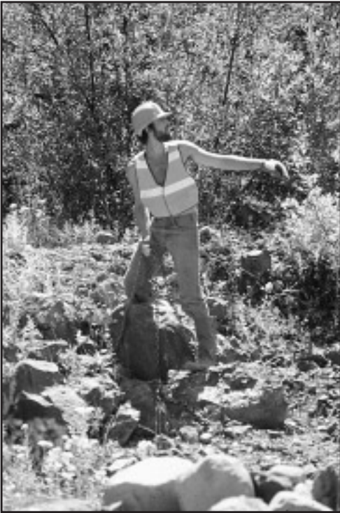
Figure 2. The collar has been placed around the base of the boulder and adjusted. Next, the load hook from the helicopter will be attached to the sling. Notice the appropriate safety gear being worn by the restoration worker.
