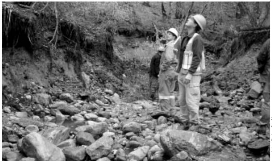
Channel erosion at Rembler Creek, October 2003.
