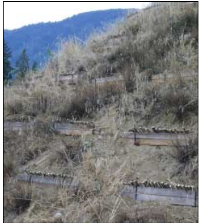
Figure 4. At this site, cedar planks were successfully utilized in modified brush layers.
