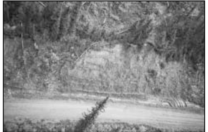
Figure 2. Hillslope stabilization along this roadway involved wattle fencing, brush layers, live silt fences, willow staking, and hydroseeding. Willow and cottonwood were the species used.
